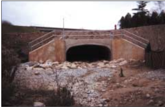
The headwaters of this former brook trout stream are buried under 3 feet of mud and rock.
