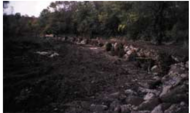
Boulders and roots line the new stream bank under the Burnhamthorpe Road bridge.
